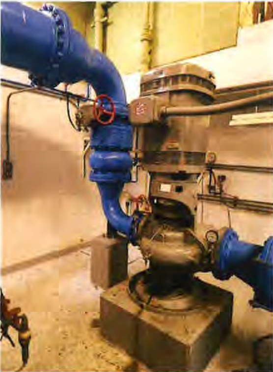
HSP5 with isolation and check valves
