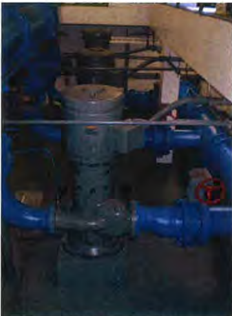
Abbey Wood Pump Station pumps
