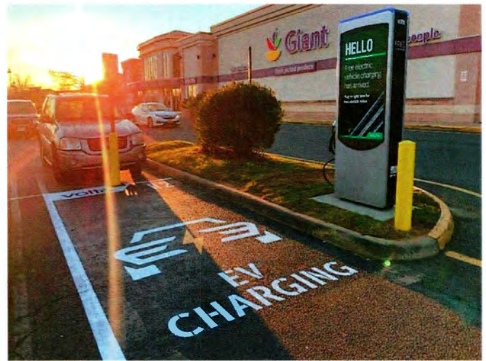
An EV-Installed parking space in Virginia (Source: Giant Foods)
