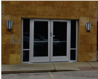
EXISTING WALL-MOUNTED ENTRANCE LIGHTS. (4) TWO TO BE RELOCATED AT TENANT ENTRANCE. MATCH WITH SIMILAR @ J-BOX ON NORTH FACE
