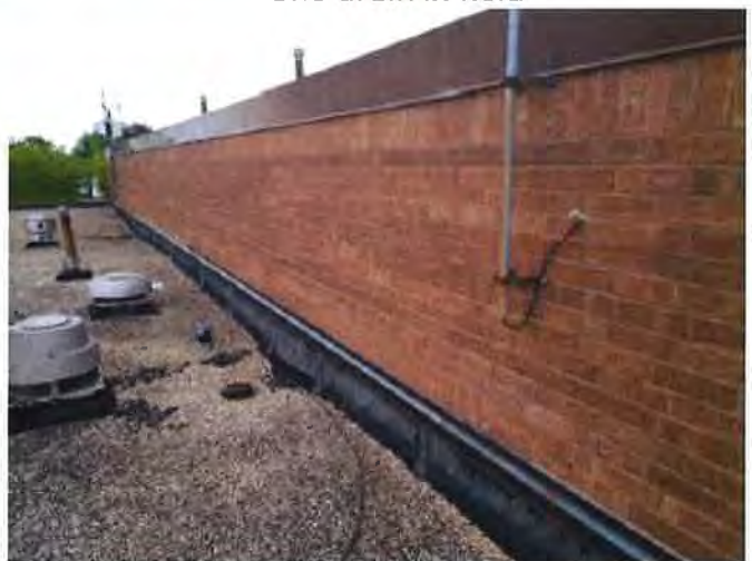
wall needs some tuck pointing
