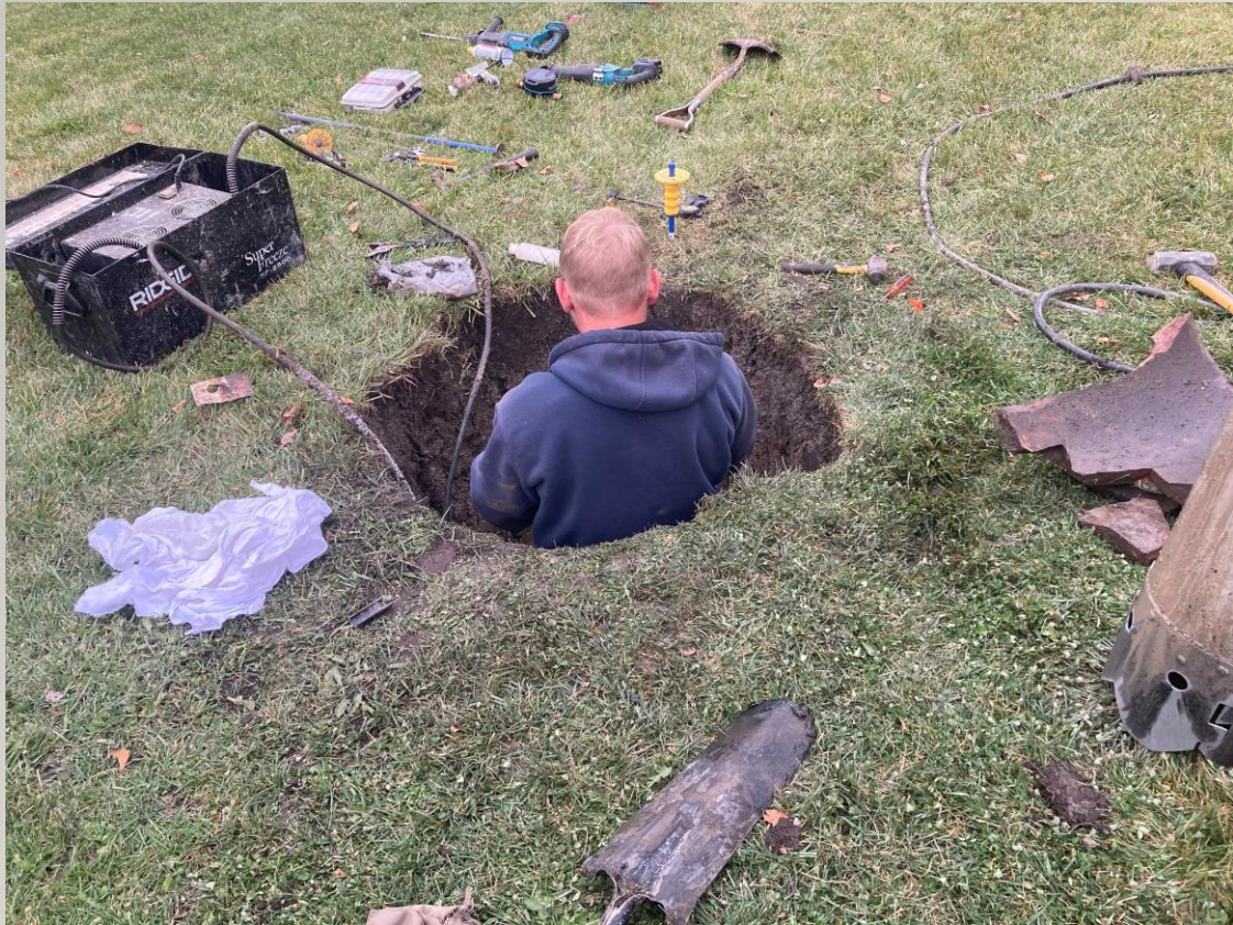
Customer Service staff use a device designed to freeze water service lines to stop water flow. Once frozen, staff can repair valves or replace water meters before returning water service.
