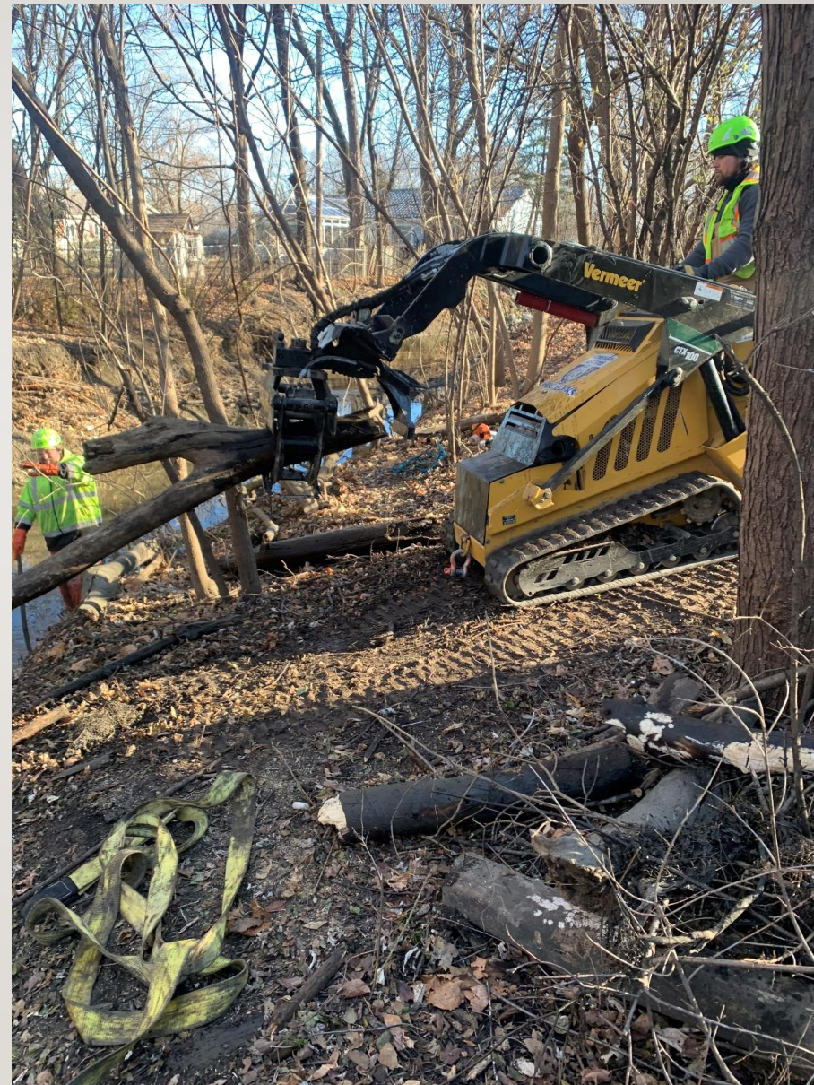
Storm Sewer Construction staff clearing debris to improve creek drainage and flow.
