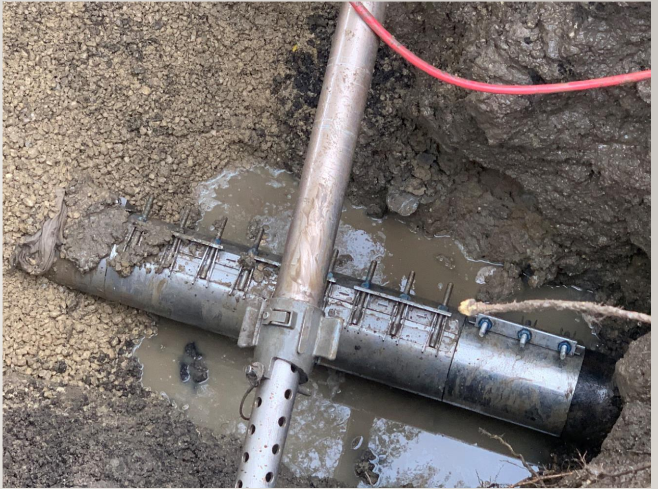
Water Construction staff excavating to install repair sleeves on a leaking water main.
