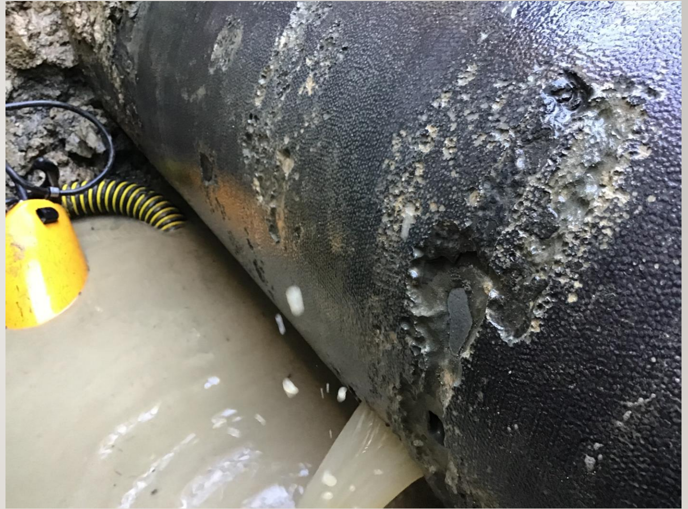
Water Construction staff using shoring to safely repair a leaking water main.
