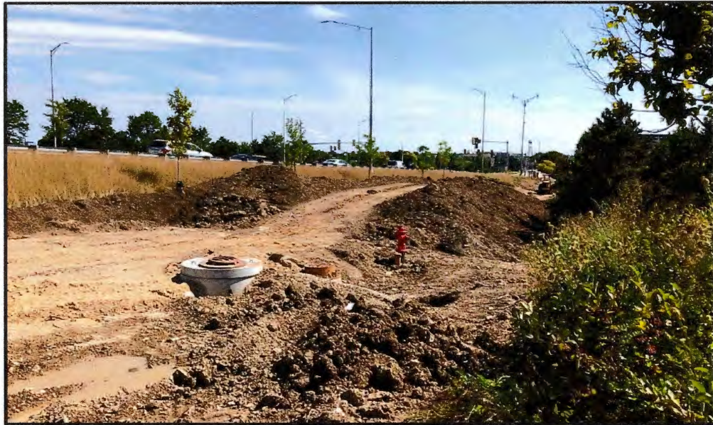
Roselle Road path construction Looking south towards Hillcrest, west side of Roselle – south of I-90
