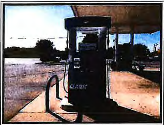
Typical Dispenser on Site
