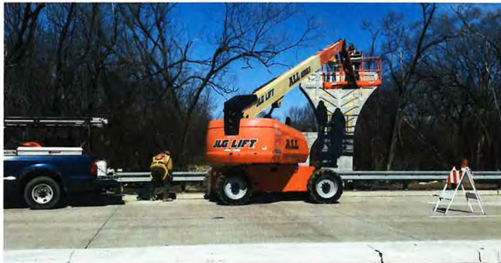
Column for Central Road Bike Bridge – Looking north from west of Roselle Road
