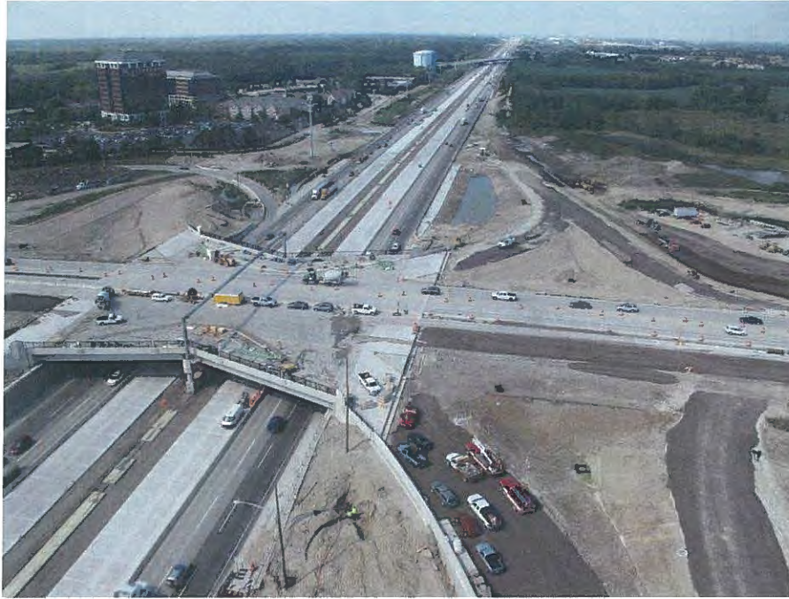
I-90 looking west at Barrington Road Grading for westbound entrance ramp in upper right
