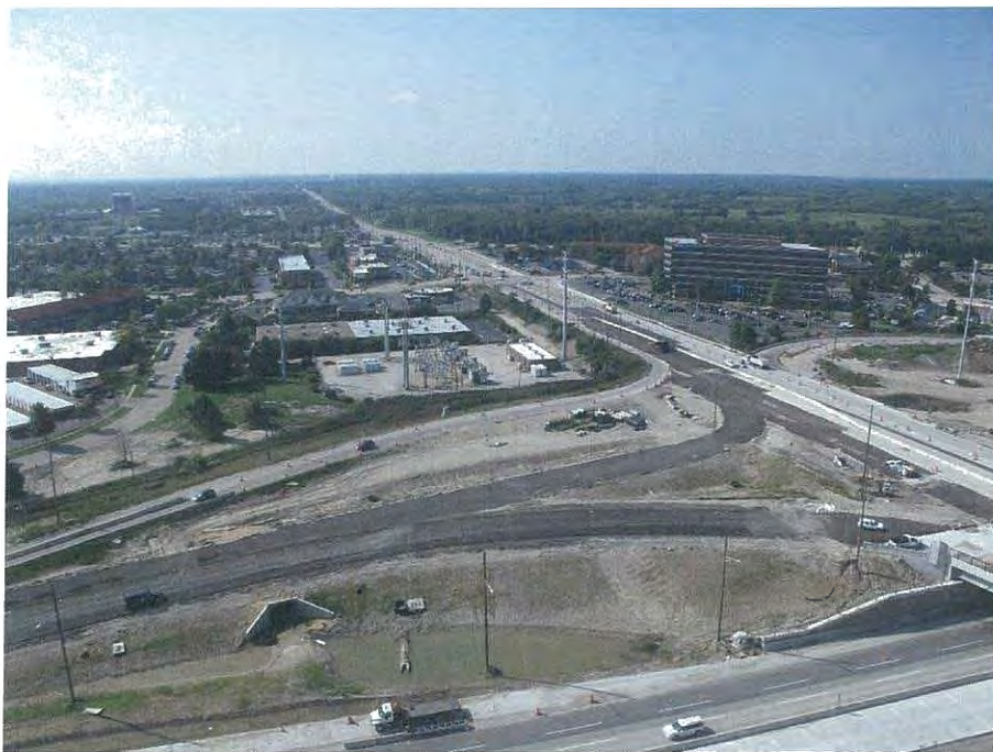
I-90 looking southwest at Barrington Road Asphalt base layer for new entrance ramp has been paved
