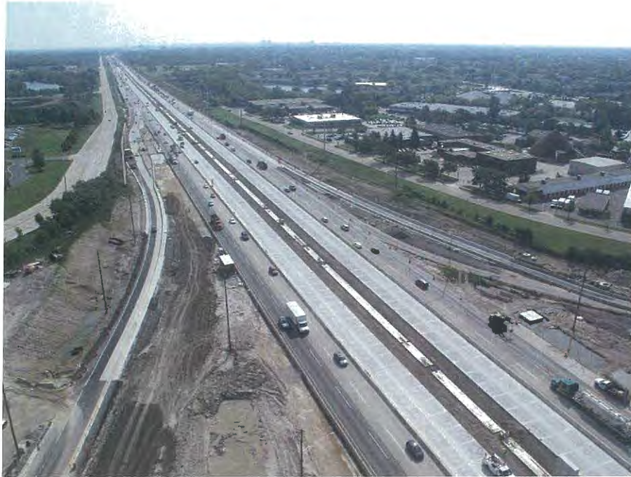
I-90 looking east from Barrington Road Base and portion of surface layer on left for new westbound exit
