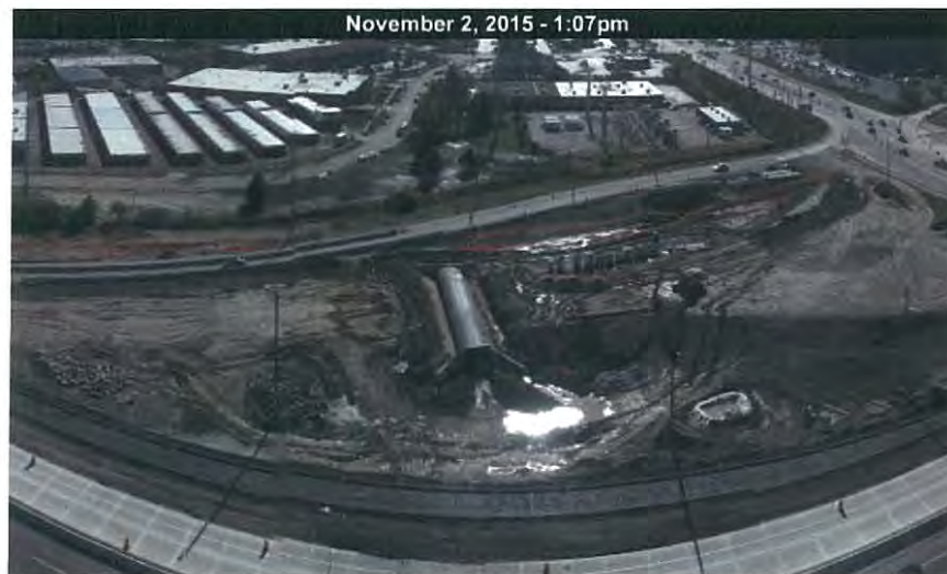
Looking southeast from I-90 at Barrington Road New eastbound entrance ramp under construction with pedestrian pass through
