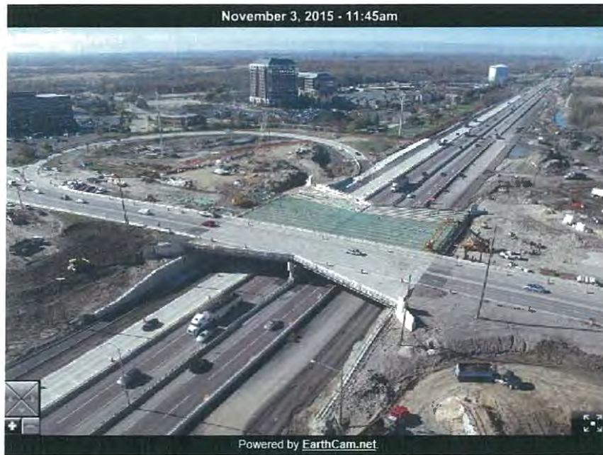
I-90 looking west at Barrington Road New half of bridge in foreground; preparing deck for concrete on west half of bridge
