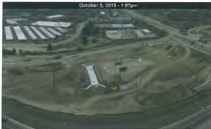
Looking southeast from I-90 at Barrington Road New eastbound entrance ramp under construction with pedestrian pass through foundation poured
