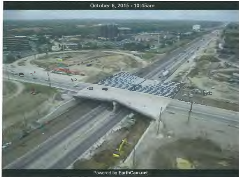
I-90 looking west at Barrington Road New half of bridge in foreground; new beams in place on west half of bridge
