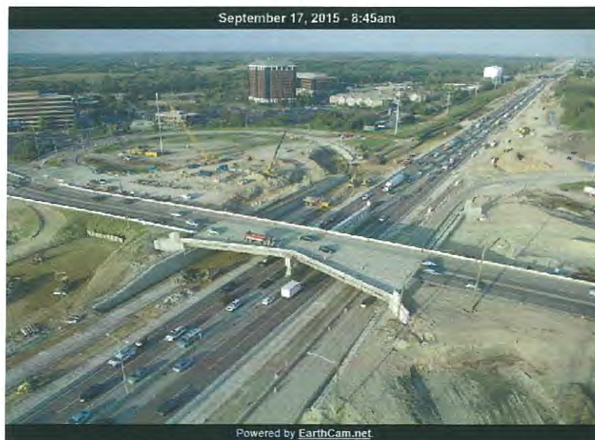
I-90 looking west at Barrington Road New half of bridge in foreground, construction underway on western half of the bridge
