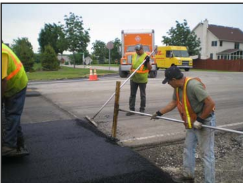
Roherssen Road is one of the many streets rehab during the 2008 Street Rehabilitation Program.
